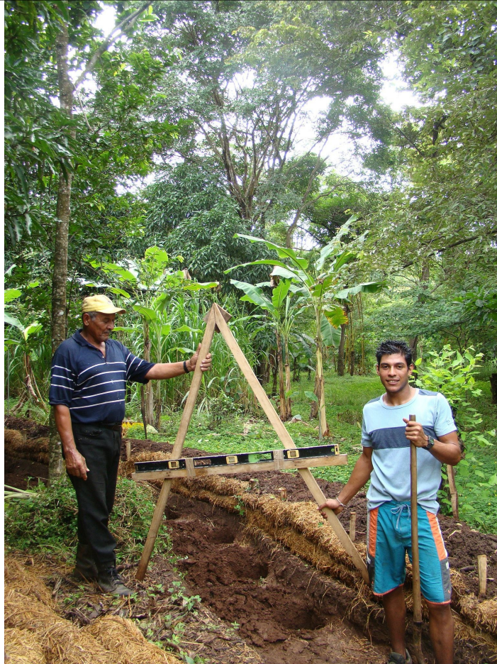
This is a more sophisticated technique of contour water spreading in a flood plain with a "fertility building trench" on the upstream side. Note all work done by hand, not backhoe. 2 men 2 days
